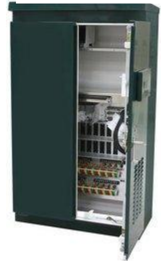
Figure 11. ATC Traffic Controller Cabinet
